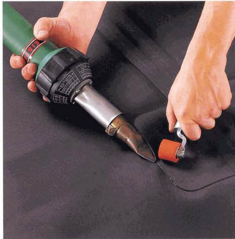
Prefabricated pipe boots, flashings and details are spliced with hot air guns. Quality control is made by means of air lance testing.
