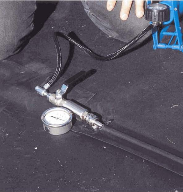
On site the Thermobond dual track seams are tested with air pressure.
